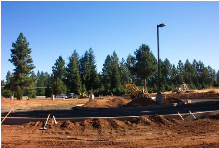
El Dorado East Natural Resources Program site in Camino: grading of new parking area completed by Doug Veerkamp General Engineering.
