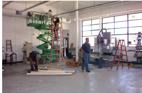
Roebbelen Construction project manager Andy Brophy oversees construction renovation of Oak Ridge High School Manufacturing Engineering Technology (MET) Lab.
