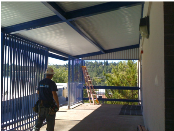
A Ski Air, Inc., employee enjoys a little shade under the new canopy installed by Phillips Steel as part of the Library and Science renovation project at El Dorado High School. Ski Air was the HVAC subcontractor on the renovation project.
